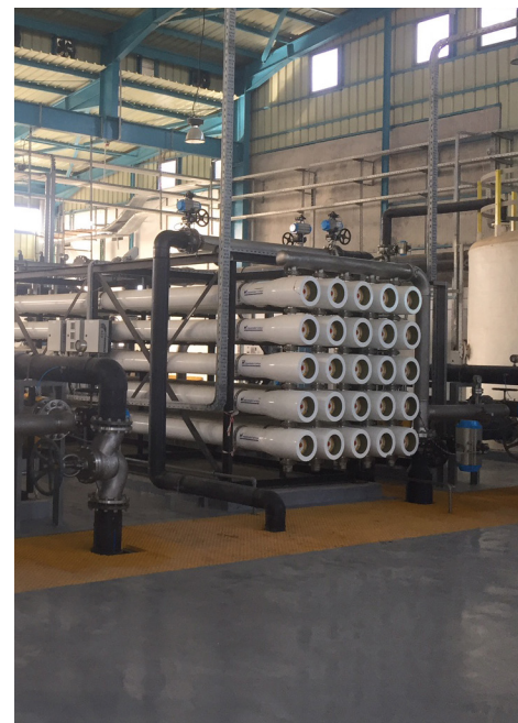
Desalination facilities of Gaza.
