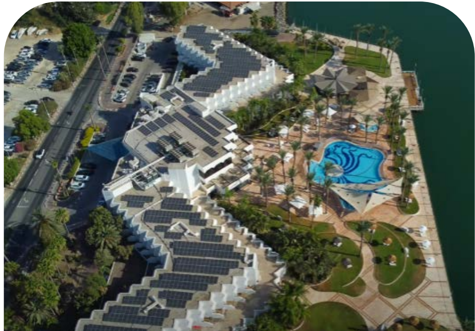
PV system on the roofs of the Gai beach hotel.
